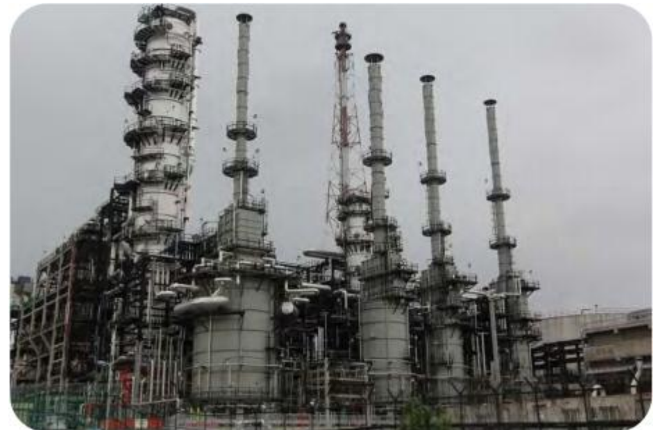
H PROJECT / SK INNOVATION, 2013' (4 Cylindrical Heaters)
