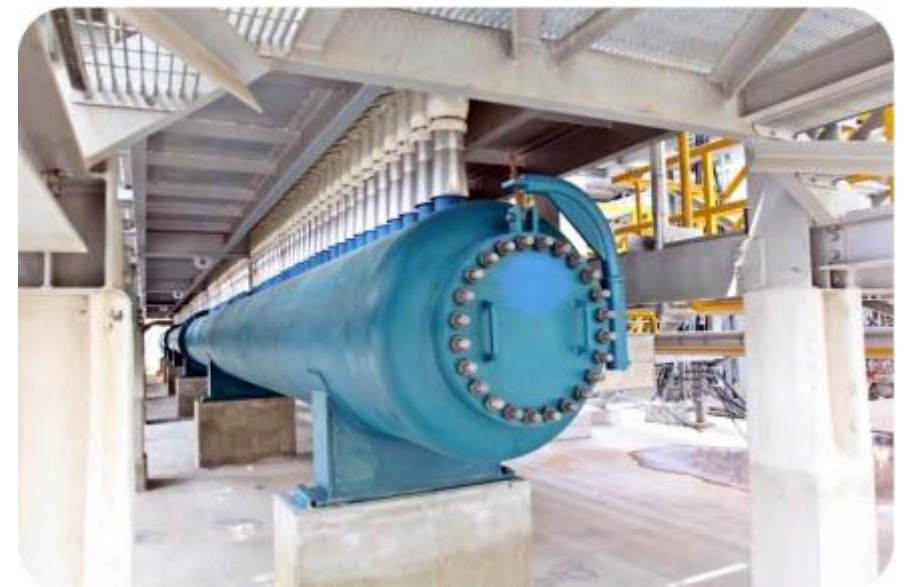
DY HYDROGEN REFORMER PROJECT / DEOKYANG 2014' (50,000 Nm 3 /h)
