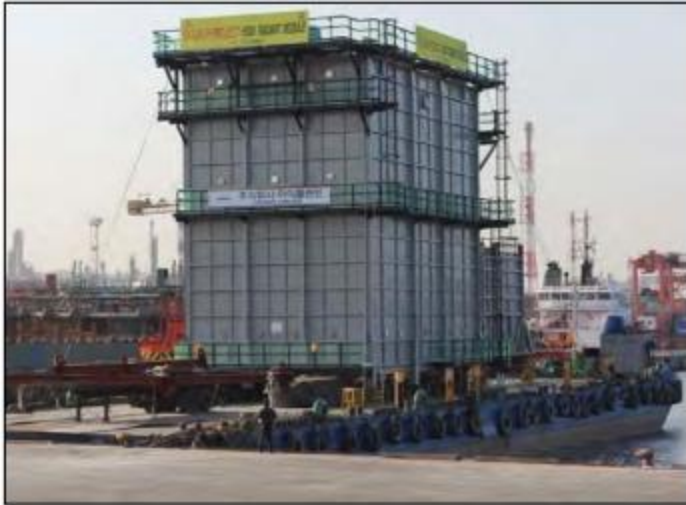
SK GAS PDH PROJECCT (2014) / SK GAS FAB. & ERECTION OF REACTOR CHARGE HEATER
