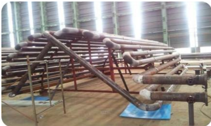
RADIANT COIL FABRICATION
