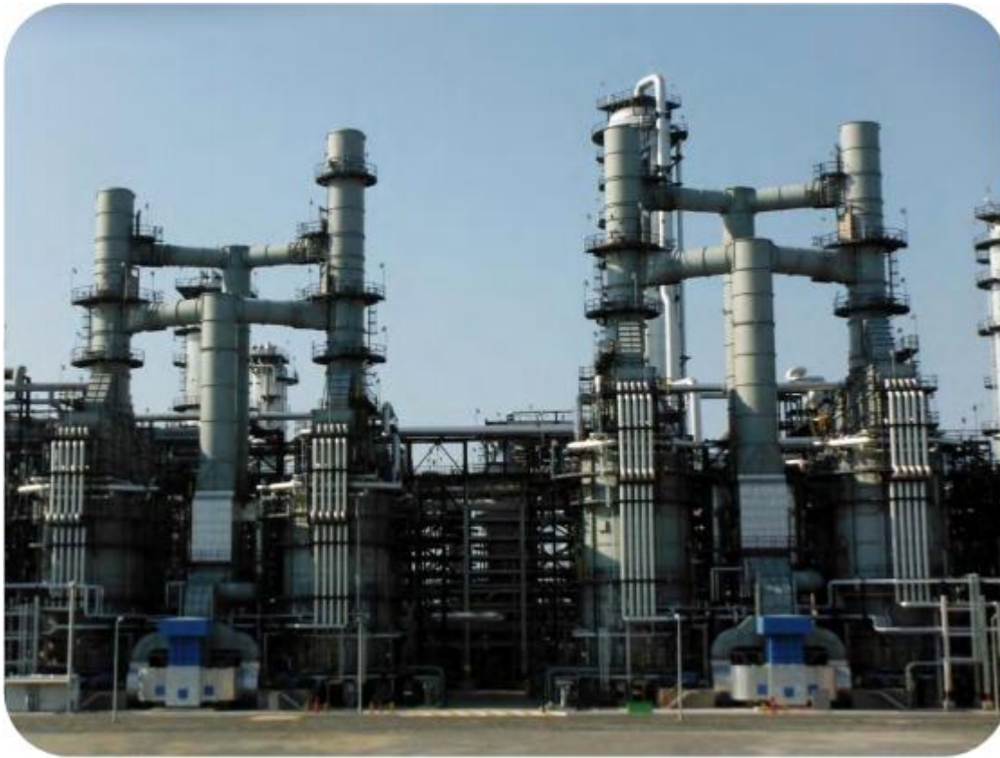
NEW PX PROJECT / SK INNOVATION, 2013' (8 Cylindrical Heaters with APH System)
