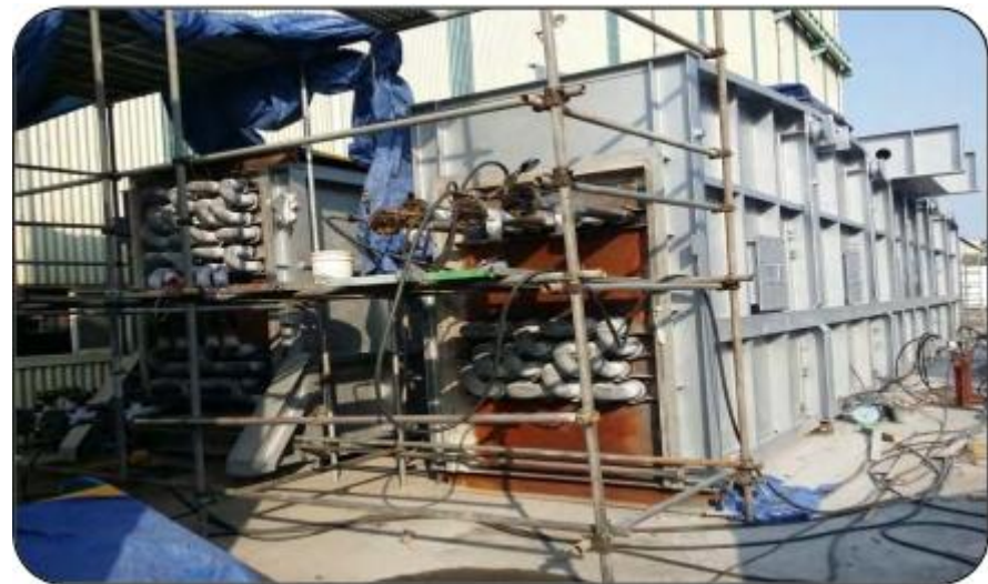
CONVECTION MODULE HYDRO. TEST
