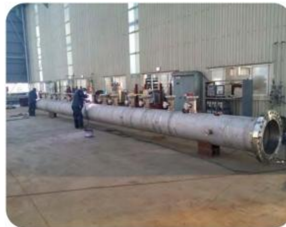
RADIANT OUTLET MANIFOLD
